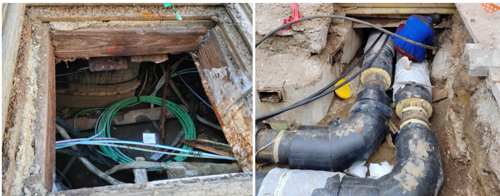
Figure 1. Use of different sewer systems for the installation of ducts and cables
